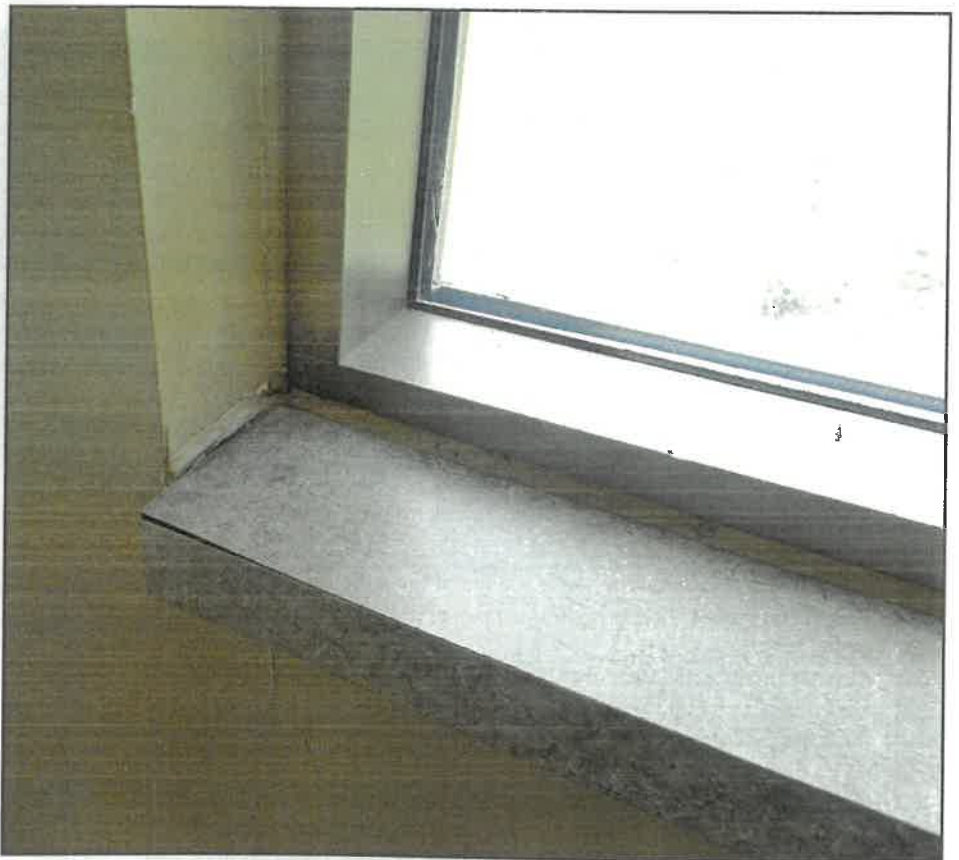
Figure 1. Visible moisture damage of the plastic laminate sills. Photo courtesy of Inspec.
